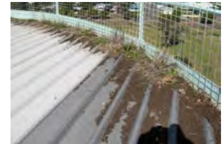
Kick rail ponding
