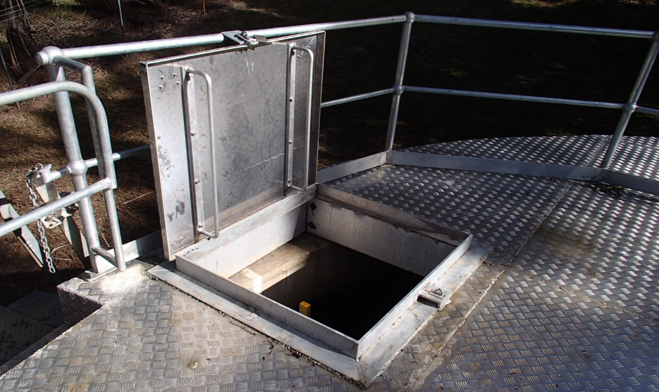
Entry hatch cover locked open with vertical hand grips in place
